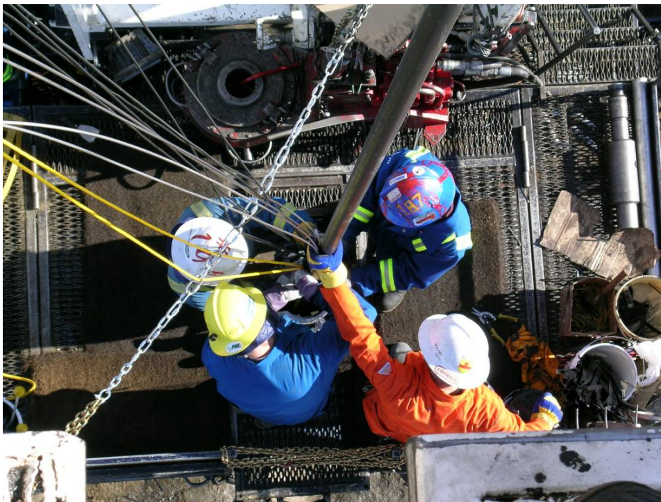
Figure 3. Detailed installation photographs showing the installation of seismic cables (yellow) alongside stainless steel fluid monitoring lines, and pressure/temperature
