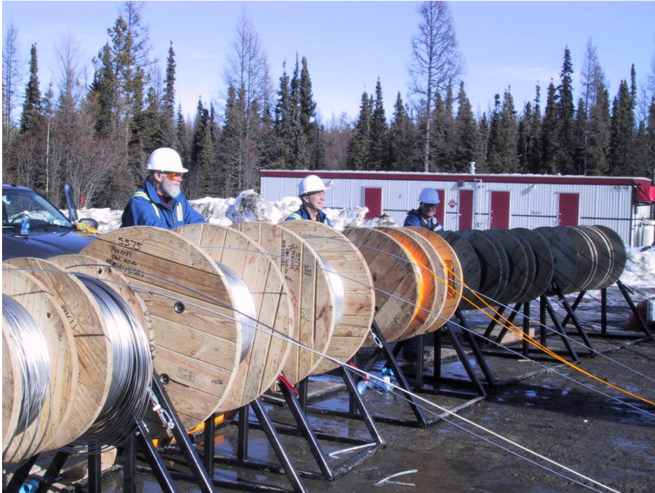
Figure 4. Cable and tubing is hand-spooled as the sensors are inserted in the borehole.
