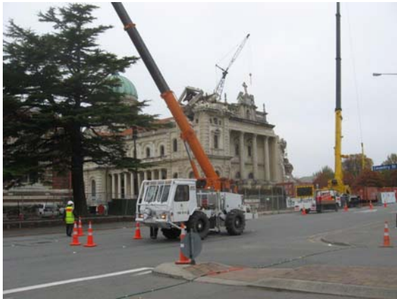
Figure 5. Source operating along Line 2, outside the heavily damaged Catholic Basilica, Christchurch.
